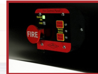
SMVS Control Panel
